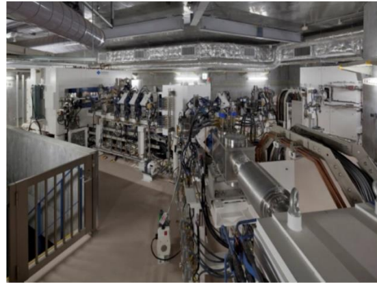
Figure 6. Appearance of proton beam transport system
